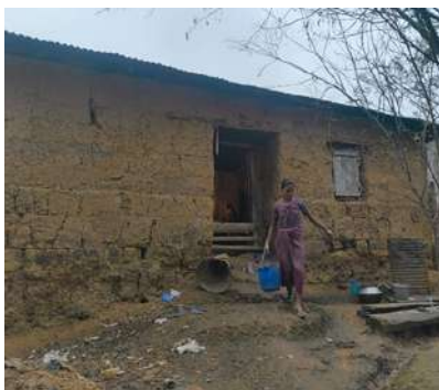
Khanda Rung's Kaccha house which used to leak during every rain posing risk of falling anytime
