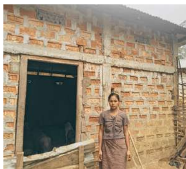
Pucca house under construction through PMAY - G with the support of Paribortan Sakhi
